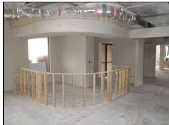
Fig. 8 Reception area with heating and air-conditioning ducts and electrical lines exposed in plenum (2' space between roof and ceiling). Top of 18" soffit above framework of future reception desk indicates final height of reception room (8'4").
